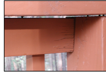
Wood Baluster shrinkage gaps
